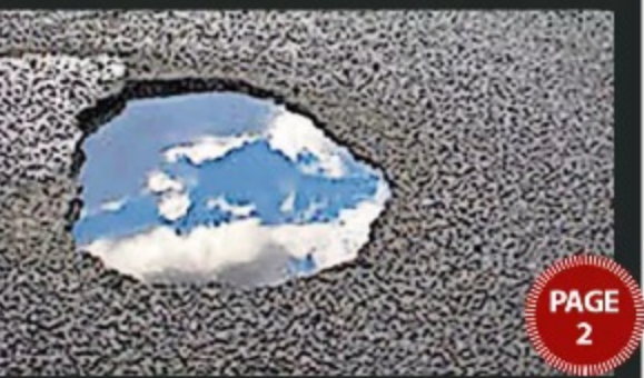
The hole truth gets worse Ayrshire motorists report more potholes on roads each year
